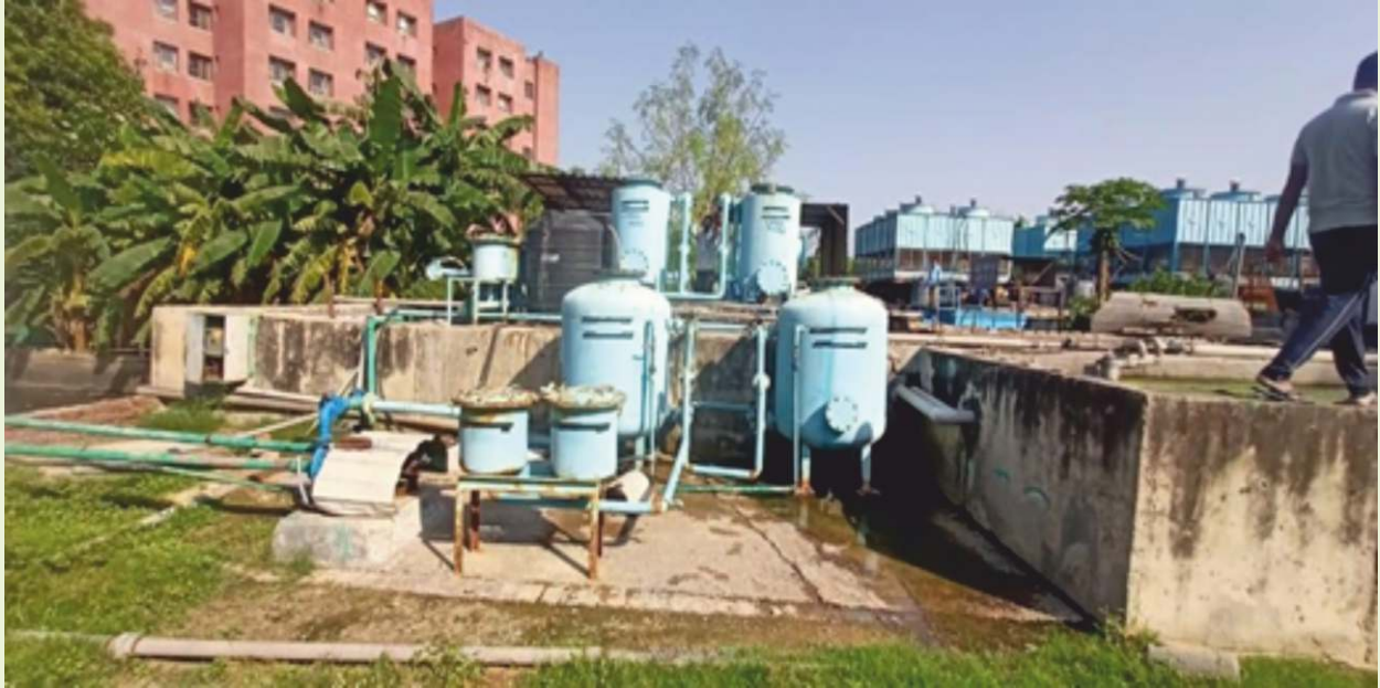
STP Plant at Amity University Haryana
