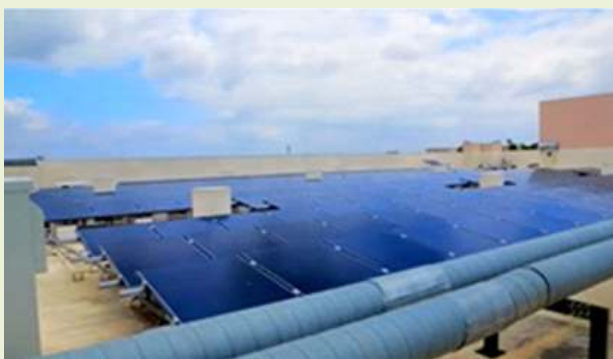
Rooftop Solar PV Plant at AUH
