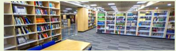
LED Lighting in Library
