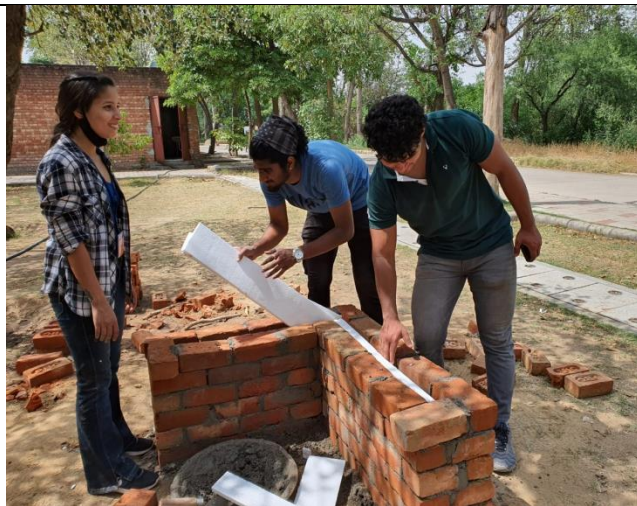
Cavity Wall -After every two layers 3 sheets of thermocol were stuffed in between the wall and butterfly ties were laid on the horizontal plane surface achieved
