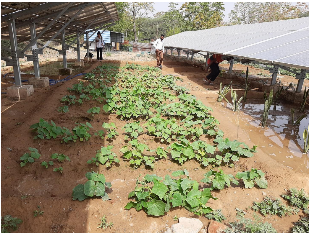
Agri-voltaic Plant at Amity University Haryana
