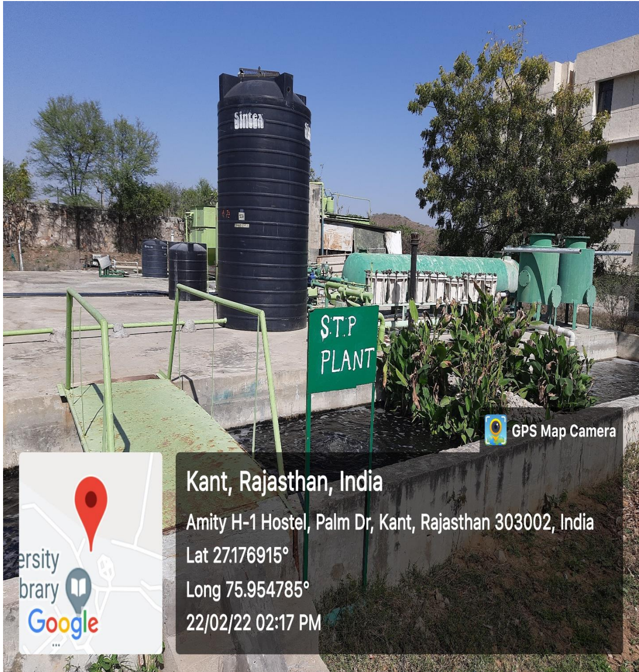
Sewage Treatment Plant (STP)
