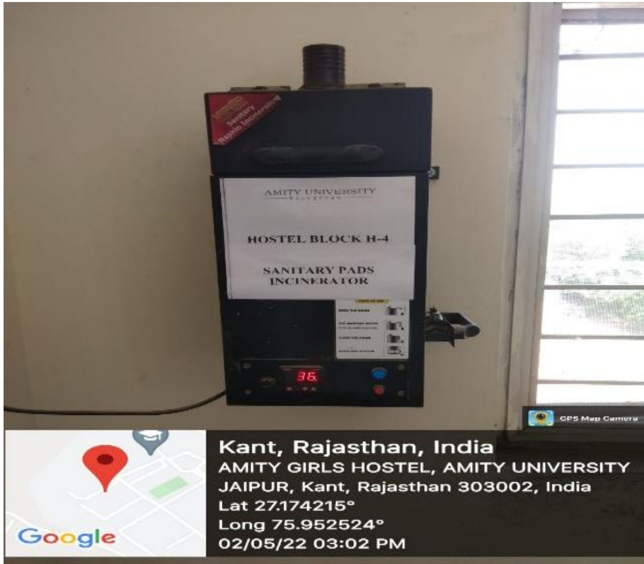
Sanitary Pads Incinerators in Girls hostel
