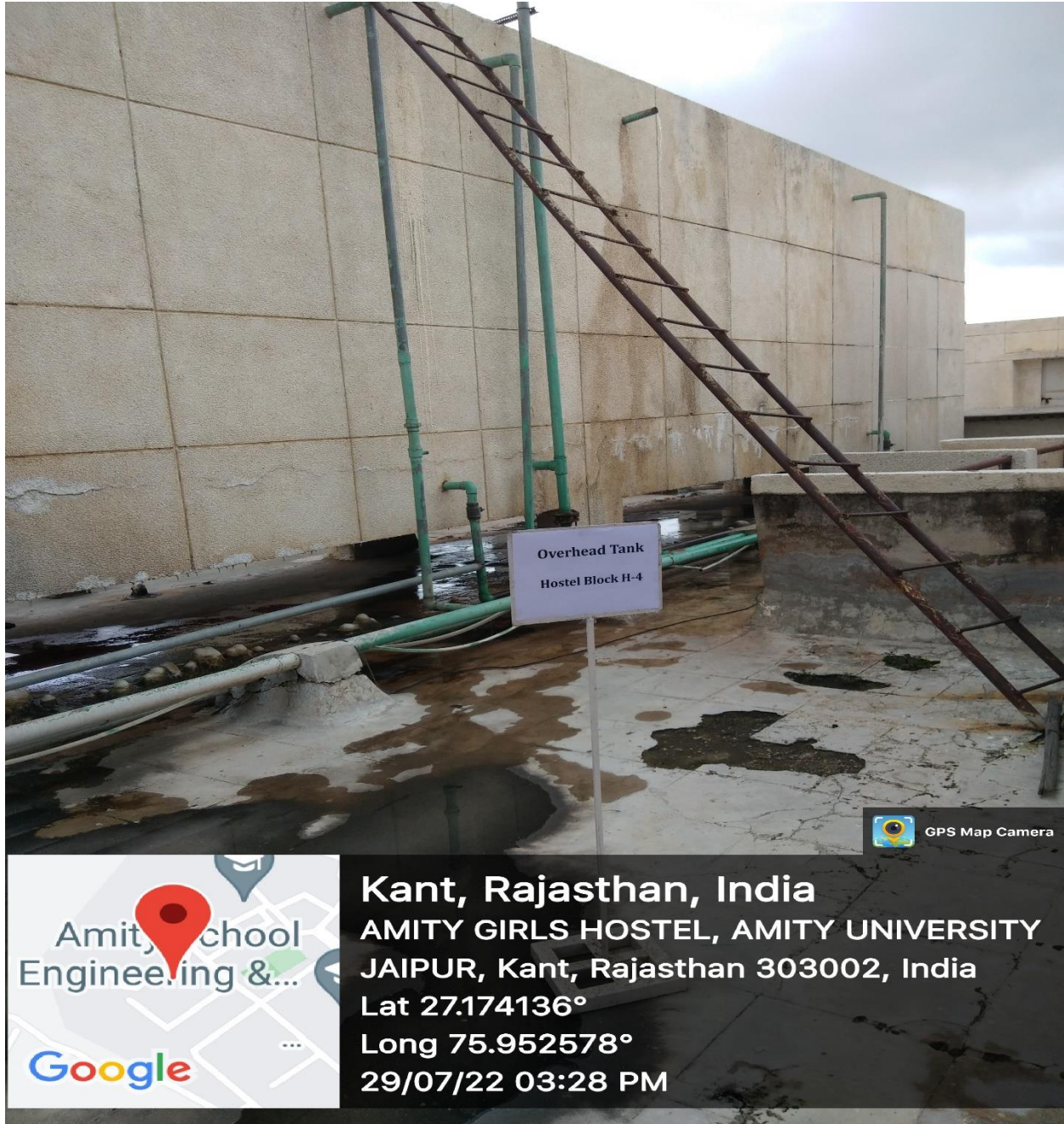
Overhead Tank Hostel Block H-4
