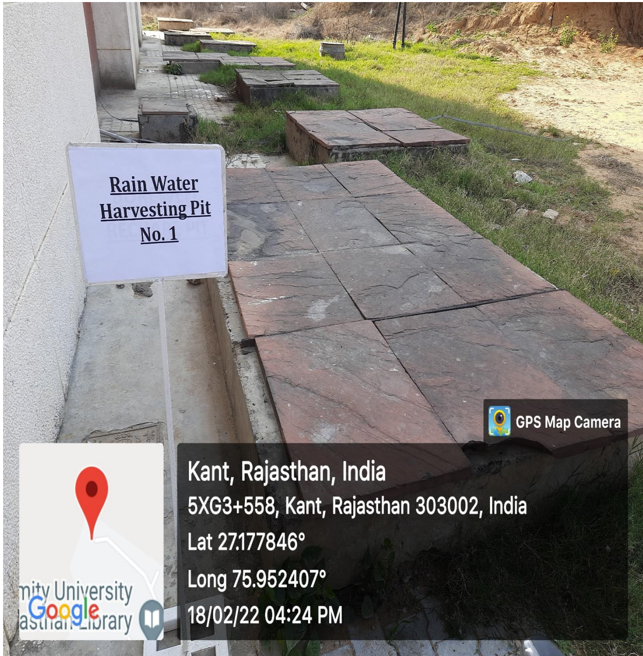
Rainwater Harvesting Pit No.-1
