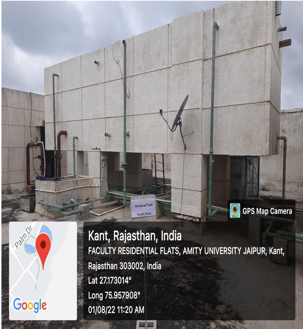
Overhead Tank Faculty Block-2
