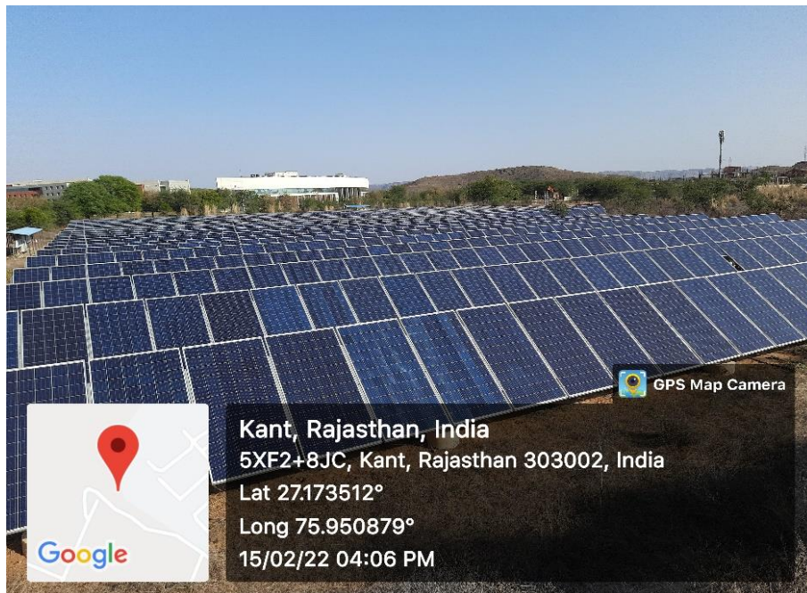
Figure-1: Solar Panel installed on roof top and ground tracker system.
