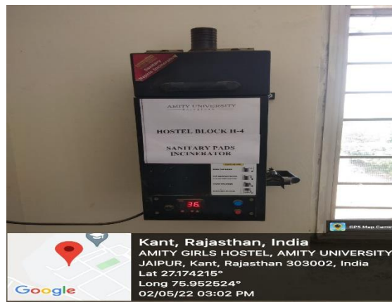
Figure-32: Sanitary Pads Incinerators available in Girls hostel (H-4).
