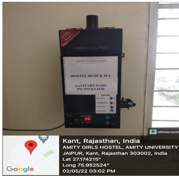
Figure-37: Sanitary Pads Incinerators available in Girls hostel (H-4).
