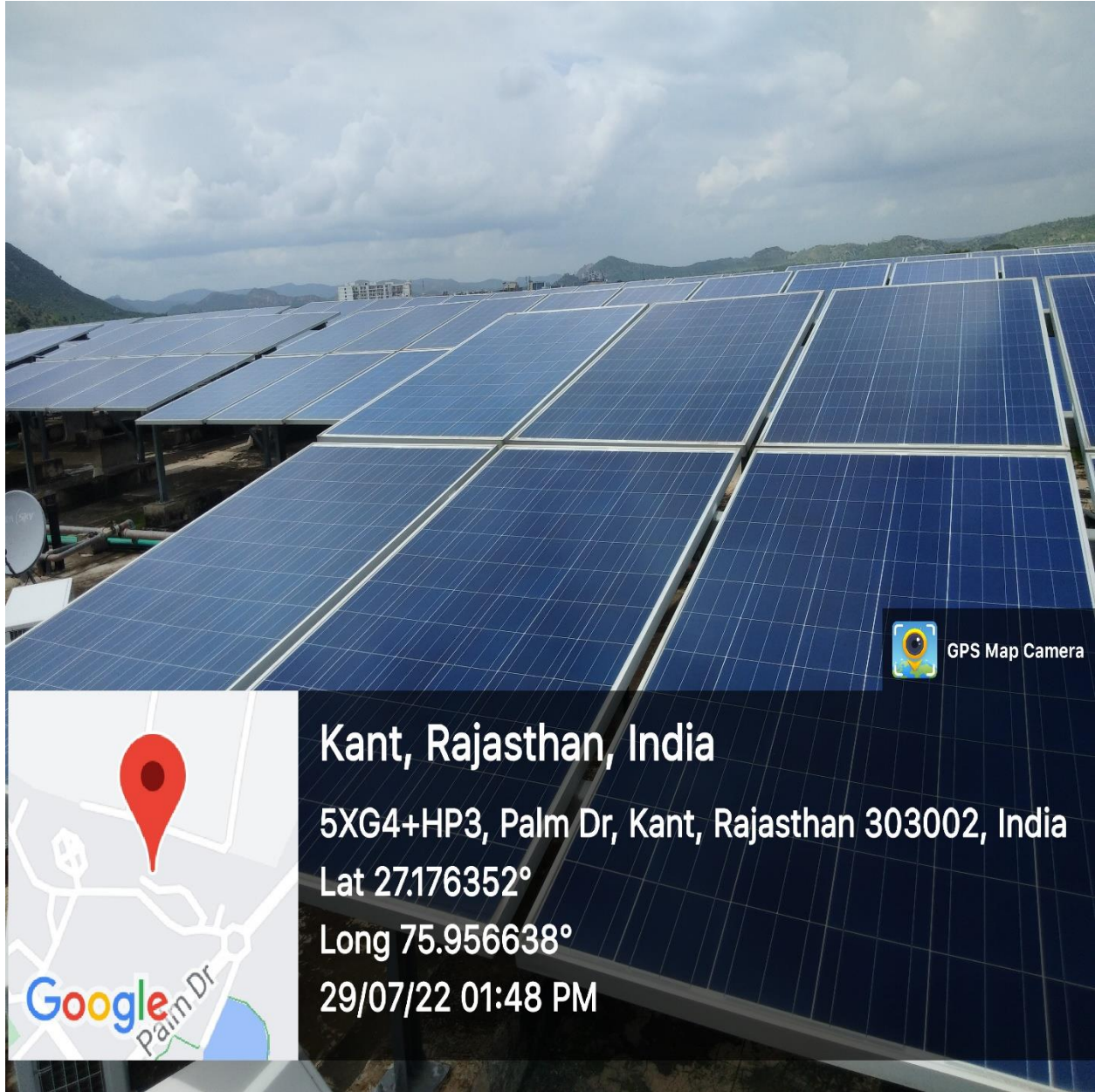
AUR Roof top Solar Panels- Academic Block A
