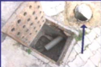
Surface Drain Pipe (Top View) Roof Top Drain Pipe (inset)
