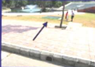
Water Collection Pit
